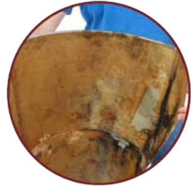
Example of polykraft use that led to corrosion of aluminum jacketing
